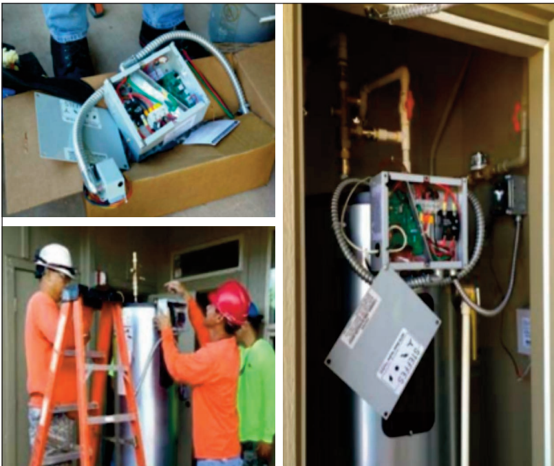
FIGURE 5: Pictures of the installation of GETS system with two-way controller (Source: presentation by Kelly Murphy of Steffes Corporation on Demand Response The Next Generation, September 23, 2015)
