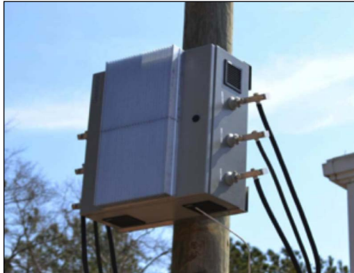
FIGURE 1: Less than 3 cubic feet wide, the 200 lb. GER is mounted on a pole.
