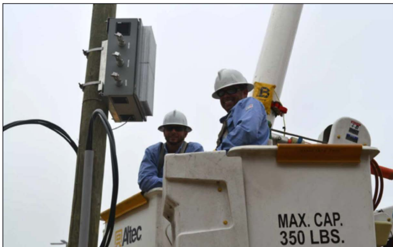
FIGURE 3: Line workers install a GER device for testing at BEMC’s warehouse.
