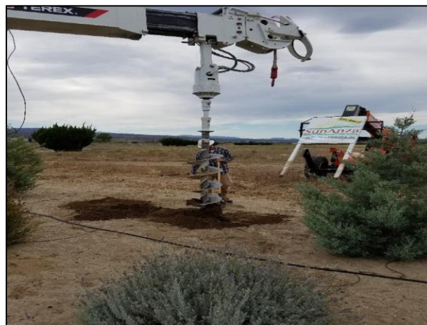
Figure 5: Santa Rosa Solar Project (Courtesy of Anza Electric)
