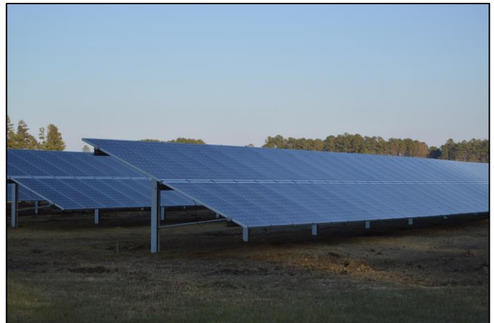
Figure 6: Solar Garden at Roanoke's Headquarters. (Courtesy of Roanoke Electric Cooperative.)
