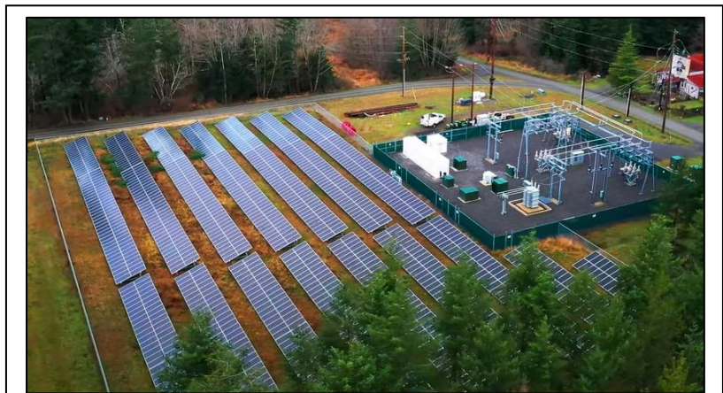
Figure 2: Decatur Island Microgrid Project
