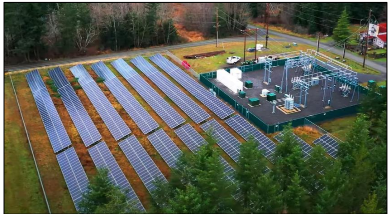
Figure 2: Decatur Island Microgrid Project
