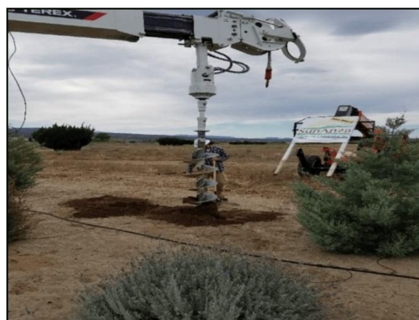
Figure 5: SunAnza Solar Project (Courtesy of Anza Electric)
