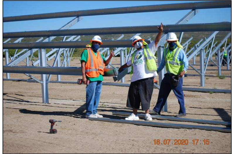
Figure 6: Anza Electric team working on the Santa Rosa Solar Project (Courtesy of Anza Electric)
