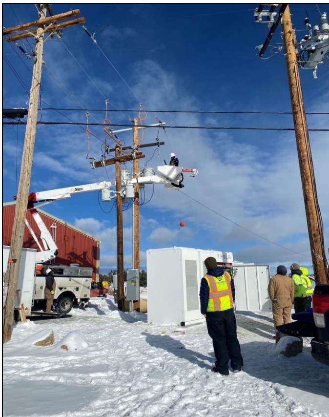
Figure 3: PVREA linemen Kevin Kelly (in bucket) and Thomas Bullock (on ground by truck) upgrading utility service for the microgrid. Image Courtesy of Poudre Valley REA.
