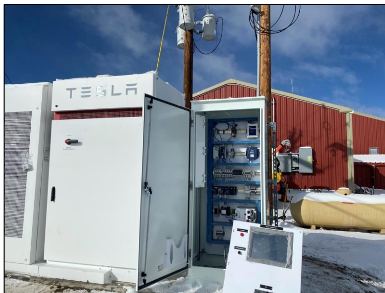
Figure 2: Installing the Encorp controller (open cabinet) next to Tesla battery outside the Red Feather Lakes fire station. Image courtesy of Poudre Valley REA.
