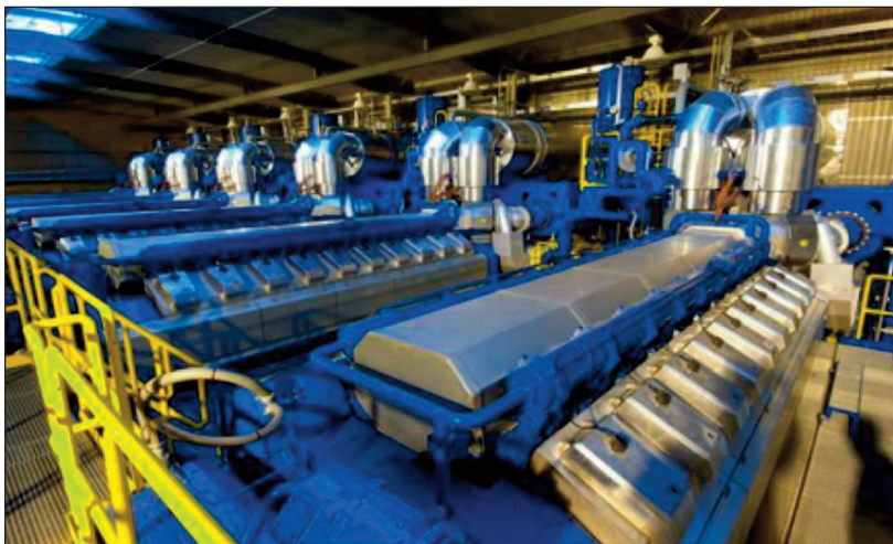
FIGURE 1: RICE units at Golden Spread's Antelope Station.
