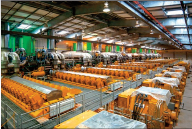
FIGURE 2: Mid-Kansas Electric's Rubart Station.
