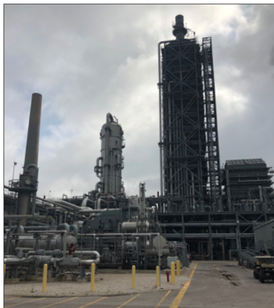
FIGURE 1: Commercial Demonstration of Absorption Technology at Petra Nova Project (Source: NRECA)
