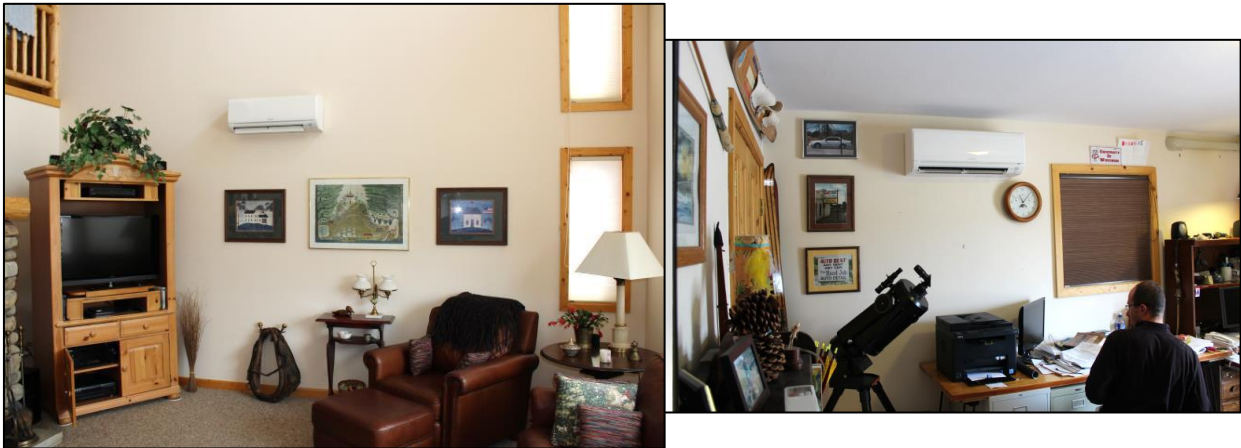
Figure 3: Indoor units installed in study home B. Left: Indoor unit 1. Right: Indoor unit 2. Photos provided by Chris Michalowski, MPE.
