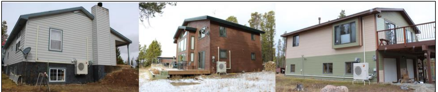
Figure 2: Outdoor units and refrigerant line conduit of ccASHP installation. Left to right: study homes A, B, and C. Photos by Chris Michalowski, MPE.
