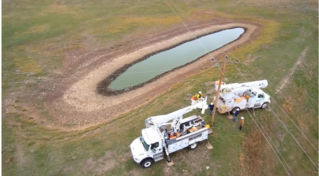
Powder River Energy line crews install avian protection devices on power lines.
