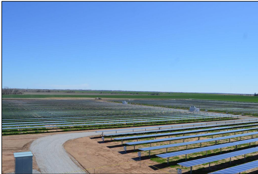
Figure 3: Western Farmers Electric Cooperative's Tuttle Solar Farm. Courtesy of WFEC.
