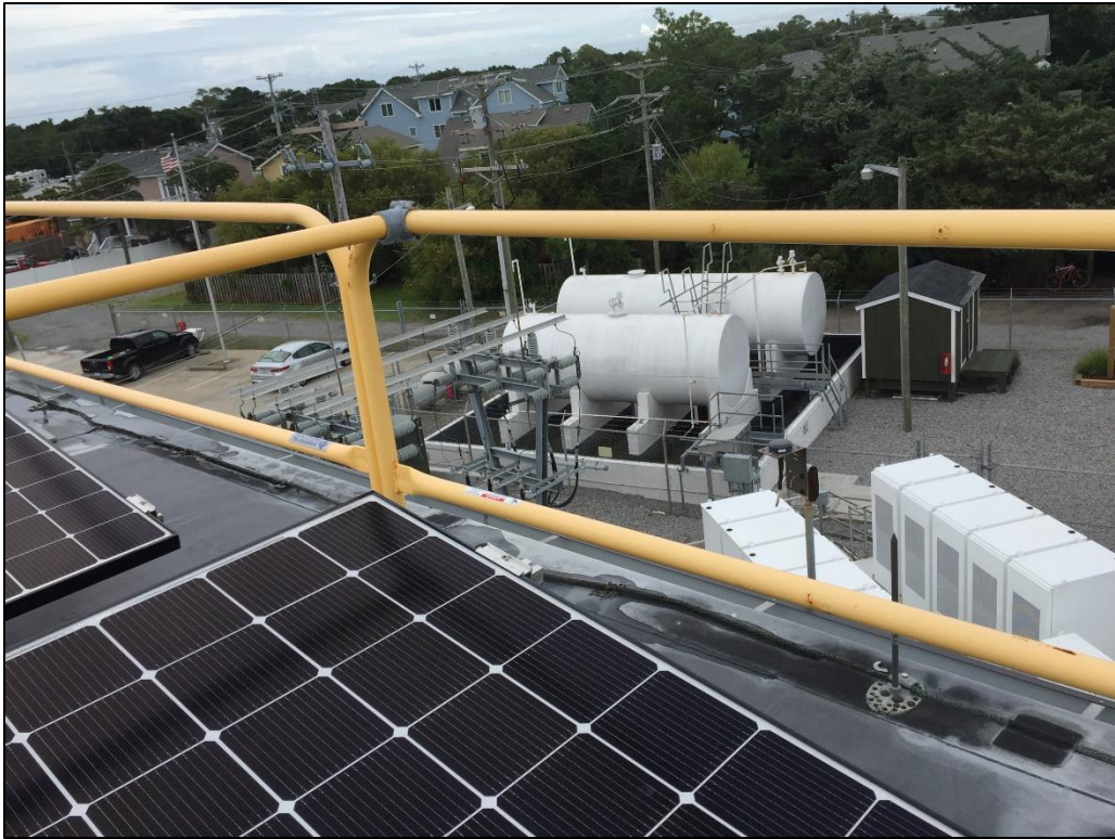
Figure 6: North Carolina EMC’s microgrid campus on Ocracoke Island includes diesel generators, battery storage, and solar generation. (Photo By: Cathy Cash, NRECA)
