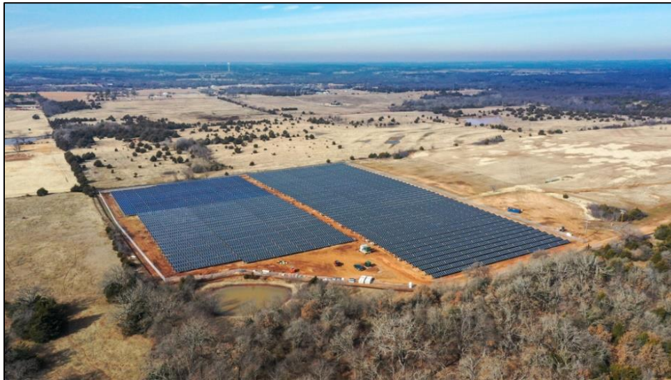
Figure 4: Oklahoma Electric Cooperative and Norman Public Schools Solar Array. Image courtesy of Oklahoma Electric Cooperative.
