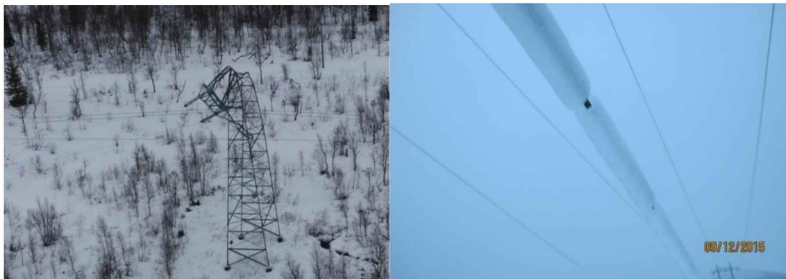
Figure 5-2: Left: Collapsed tower number 96. Right: Remaining ice on the broken earth wire, three days after the incident.
