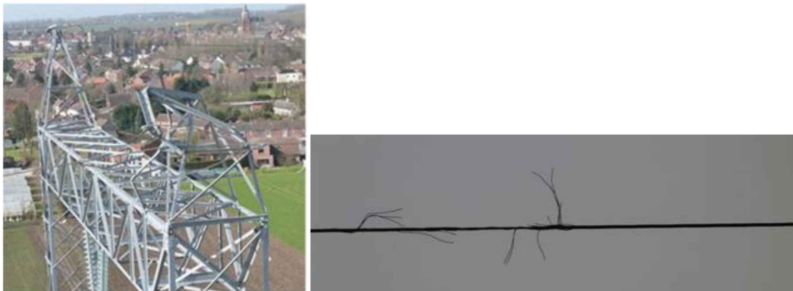
Figure 3-2: Damage to a tower and earth wire caused by the wet snow storm in Lille, 5 March 2012 (Photos: RTE, France).
