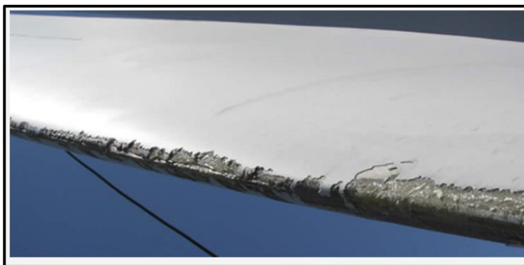
Figure 2: Wind Turbine Blade Erosion
