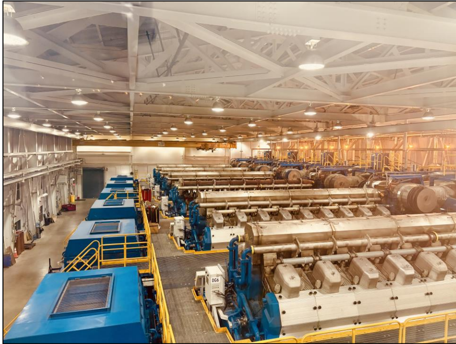
Figure 8: Matanuska Electric Association's Wartsila Engine Site
