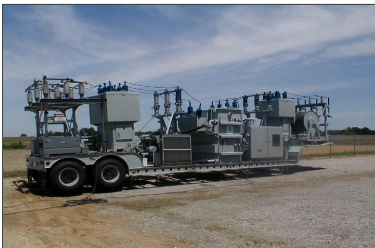
Figure 1: Example of a Mobile Substation (Courtesy of NCEMC)
