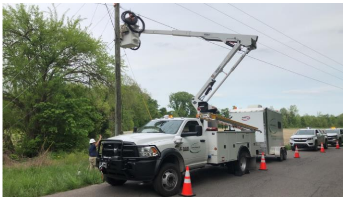
Figure 2. Crew installing a fiber splitter cabinet in the Pleasant Grove area outside of Brownstown, Indiana. Photo courtesy of Jackson Connect, LLC.
