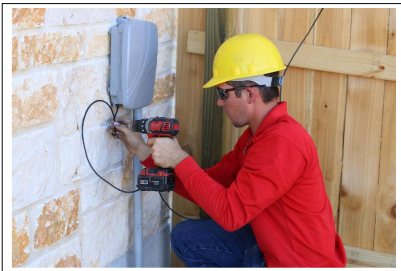
Figure 2. GVEC employee installs a network interface device (NID) on the outside of a subscriber's home. Photo courtesy of GVEC.
