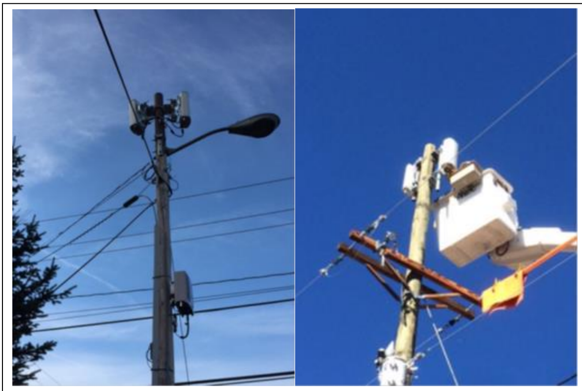
Figure 4. Small cell and outdoor DAS installations. Photos courtesy of RidgeLink, LLC.
