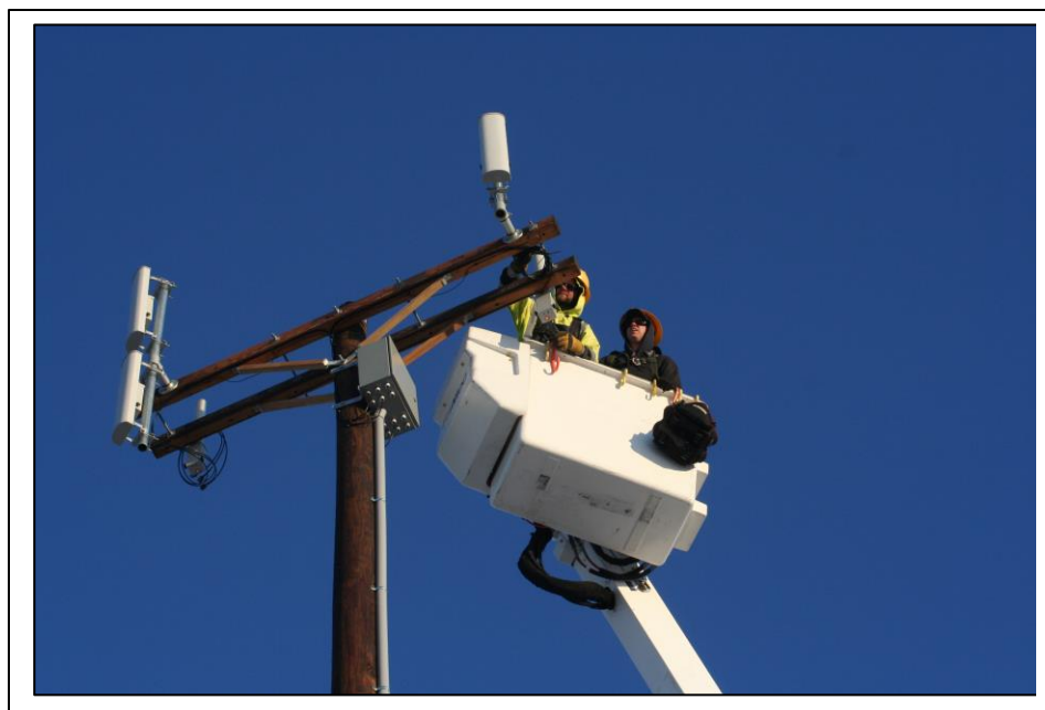
Figure 2. Workers installing wireless broadband equipment on pole Photo courtesy of Allamakee-Clayton Electric Cooperative
