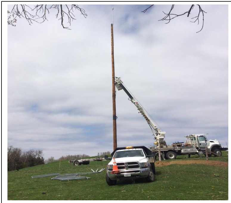
Figure 3: AC Skyways crew installs a 70-foot pole for a new micro-repeater site Photo courtesy of Allamakee-Clayton
