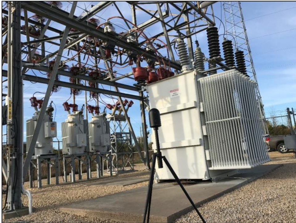
Figure 4. Digital camera on tripod scanning a substation. Image courtesy of Jo-Carroll Energy.
